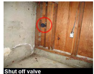
Shut off valve
